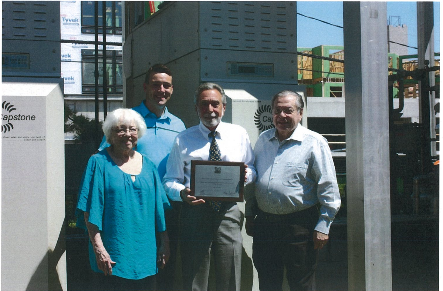
Photo 1: (L-R) Great Neck Water Pollution Control District Commissioner Deena Lesser, Superintendent Christopher Murphy, Commissioner Steve Reiter and Chairperson Jerry Landsberg stand in front of the District's microturbine cogeneration facility, for which the District was recently awarded the ACEC New York Engineering Excellence Platinum Award. The District received this prestigious award for pioneering sustainable technology by using methane waste gas in a sustainable, efficient and economical way.
